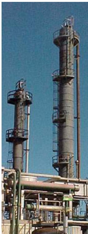
Figure 2 – Organic Acid Separation Train, Celanese, Pampa, TX
