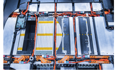
FIGURE 18 EV Battery with orange fuses, connectors and cabling attached.
