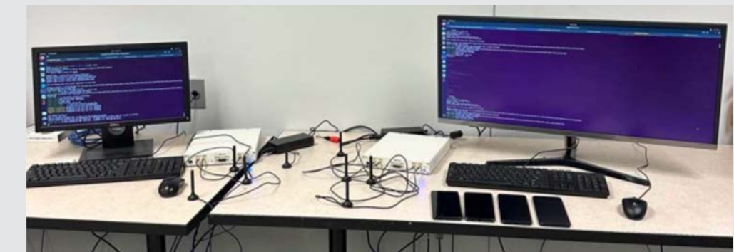
FIGURE 1. AN OAIC TESTBED PLATFORM AT GMU PROVIDES A 5G O-RAN SYSTEM WITH ONE BS AND FIVE UES (ONE SDR-BASED UE AND FOUR COTS UES).
