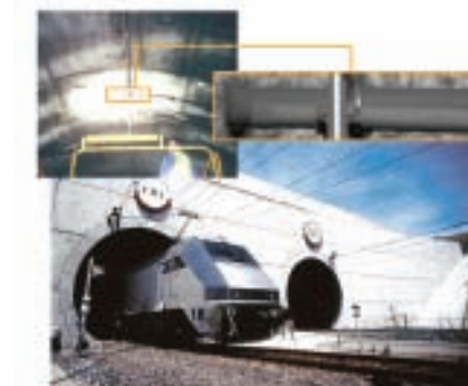
The Channel Tunnel uses NI LabVIEW software and vision products to measure more than 100 km of electrical cabling.
