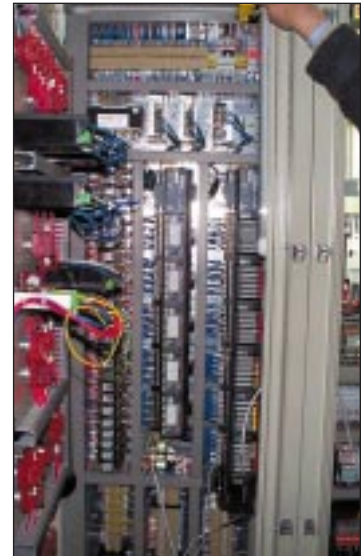
Detail of the QCC where the FieldPoint system is installed.
