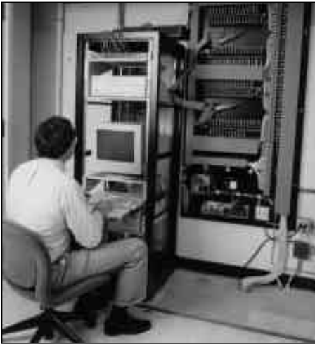
Low-speed computer room monitors collect measurements of power consumption, temperature, and humidity, sending them to a data manager.
